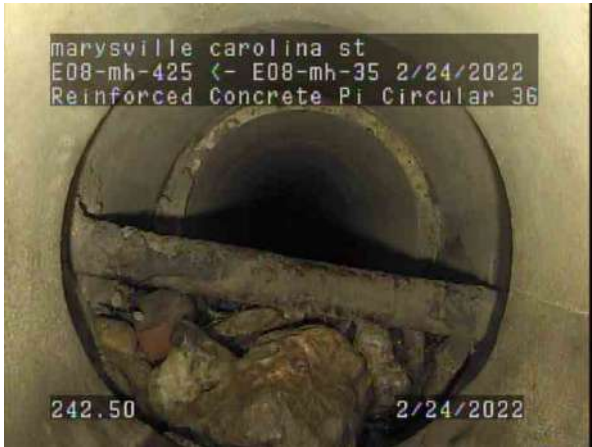
31, 00:11:14, 242.50ft Obstruction Rocks, 25% of cross sectional area from 4 o'clock to 9 o'clock
