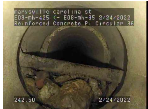
32, 00:11:27, 242.60ft Miscellaneous Survey Abandoned / stopped due to cross bore
