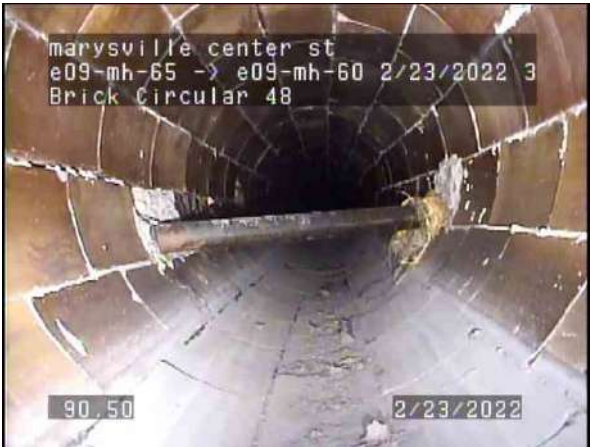
7, 00:04:16, 90.40ft Hole Void Visible from 8 o'clock to 9 o'clock
