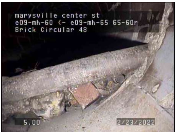
3, 00:02:06, 5.00ft Obstruction Brick or Masonry, 10% of cross sectional area from 5 o'clock to 7 o'clock
