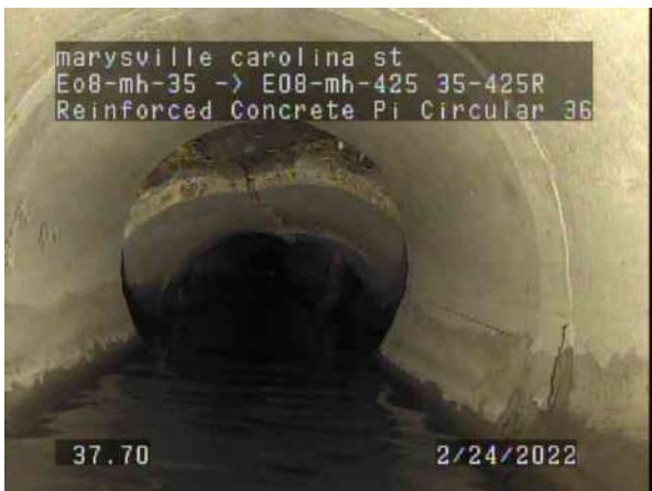
9, 00:04:01, 37.70ft Fracture Longitudinal at 4 o'clock, within 8 inch
