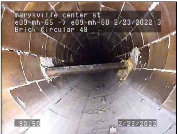
9, 00:04:26, 96.30ft Obstruction Intruding Through Wall, 20% of cross sectional area from 4 o'clock to 8 o'clock
