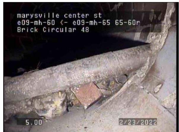
4, 00:02:16, 5.00ft Obstruction Intruding Through Wall, 20% of cross sectional area from 4 o'clock to 8 o'clock
