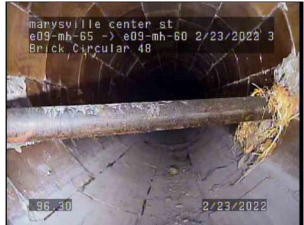
8, 00:04:51, 96.00ft Roots Medium Barrell from 3 o'clock to 4 o'clock, 10% of cross sectional area
