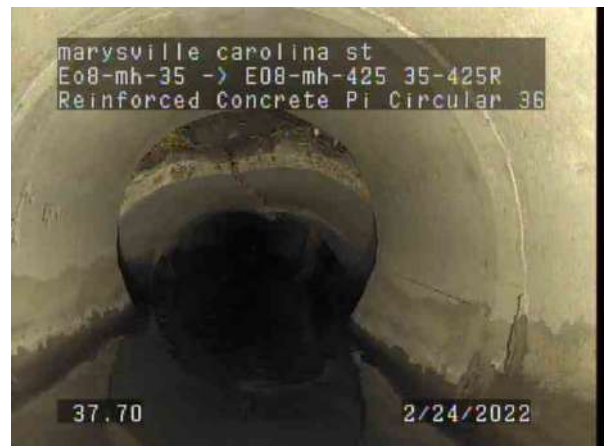
10, 00:04:29, 37.70ft Miscellaneous Survey Abandoned / collapse pipe
