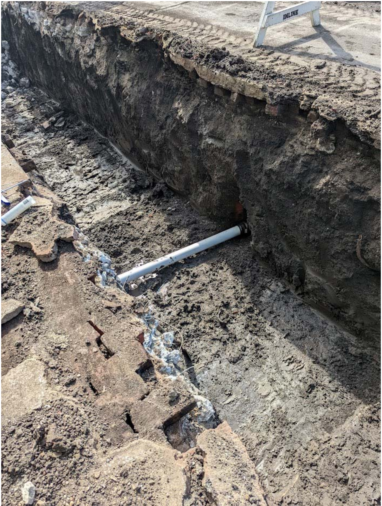
Replaced sanitary sewer service line that was crushed by the existing storm sewer.
