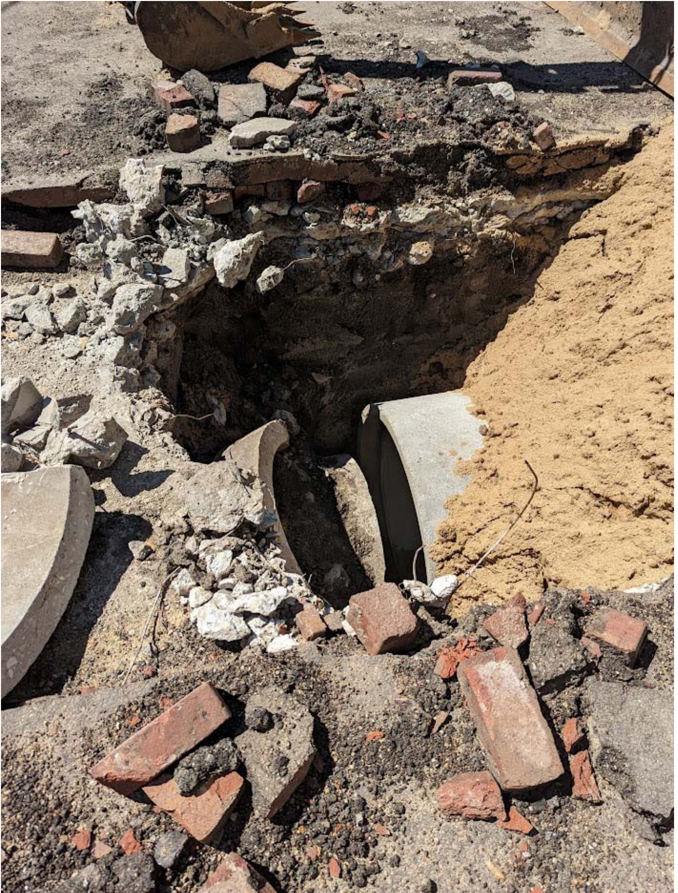
First section of new pipe is in the ground and covered with sand. New pipe next to existing pipe.
