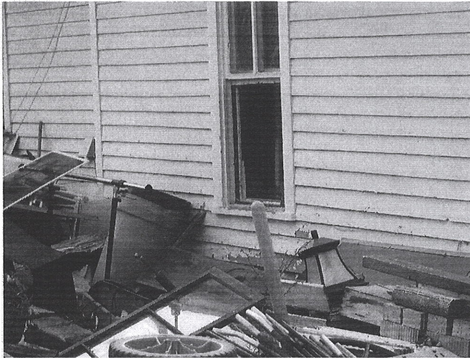
Broken Window on east side of house
