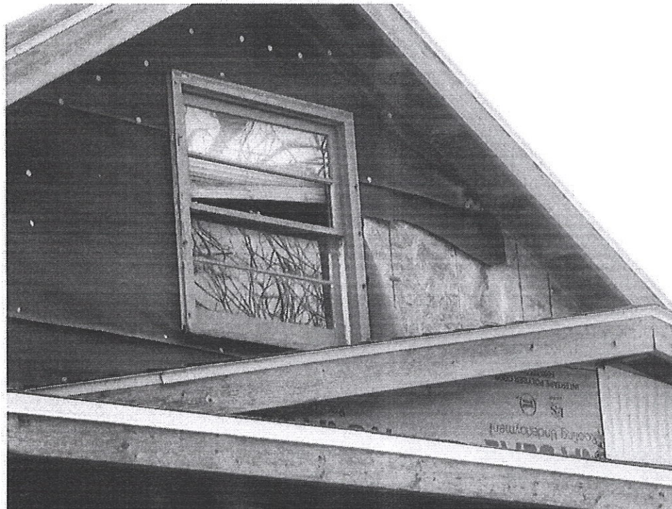
Broken window and missing siding north side of house
