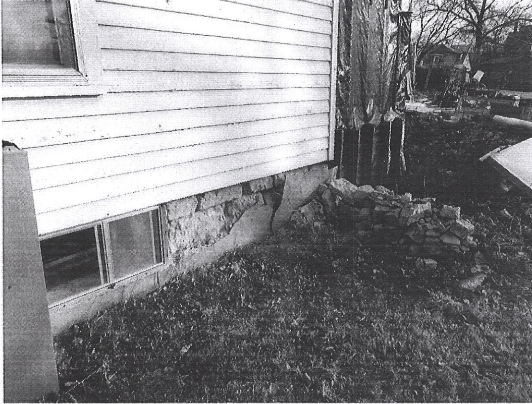
Southwest corner of the house. Mortar is missing between limestone block
