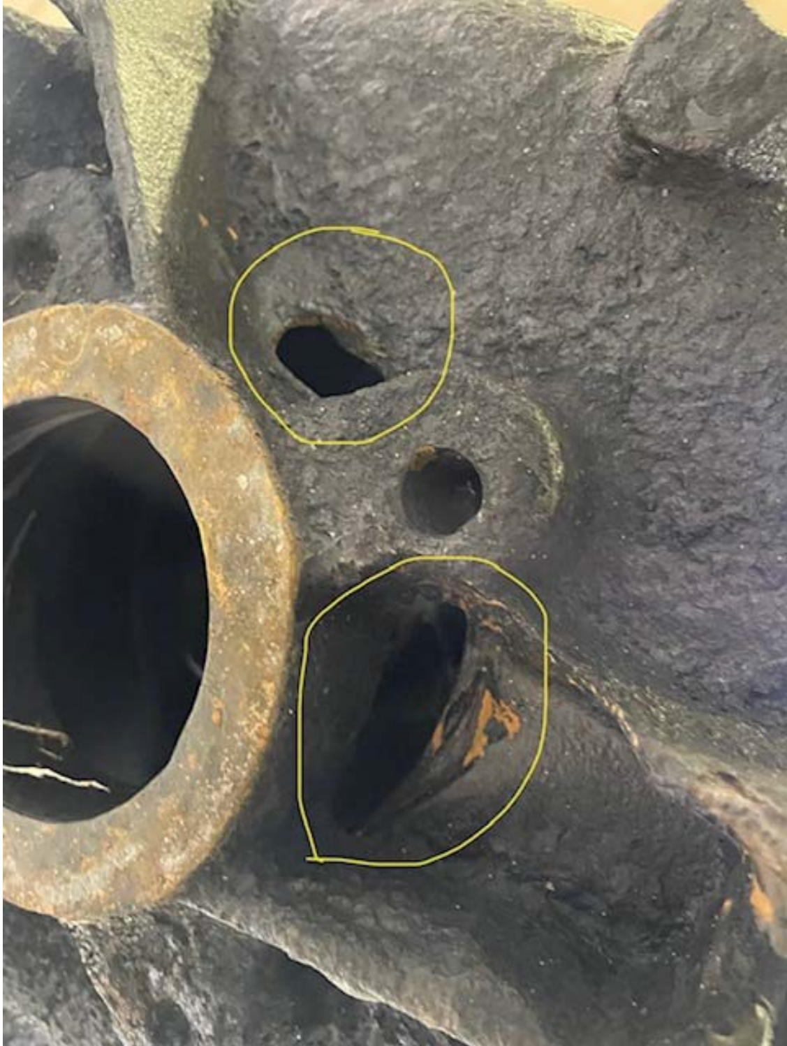
Lift Station #3 Pump with holes worn in housing
