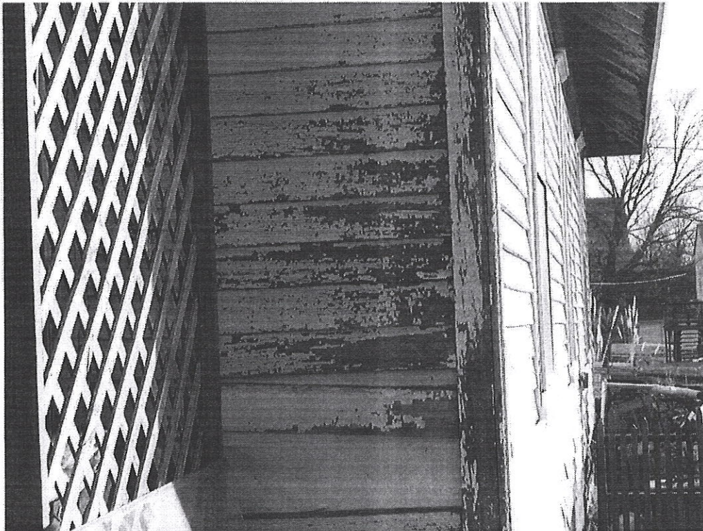
Paint peeling on North side of house and under eaves
