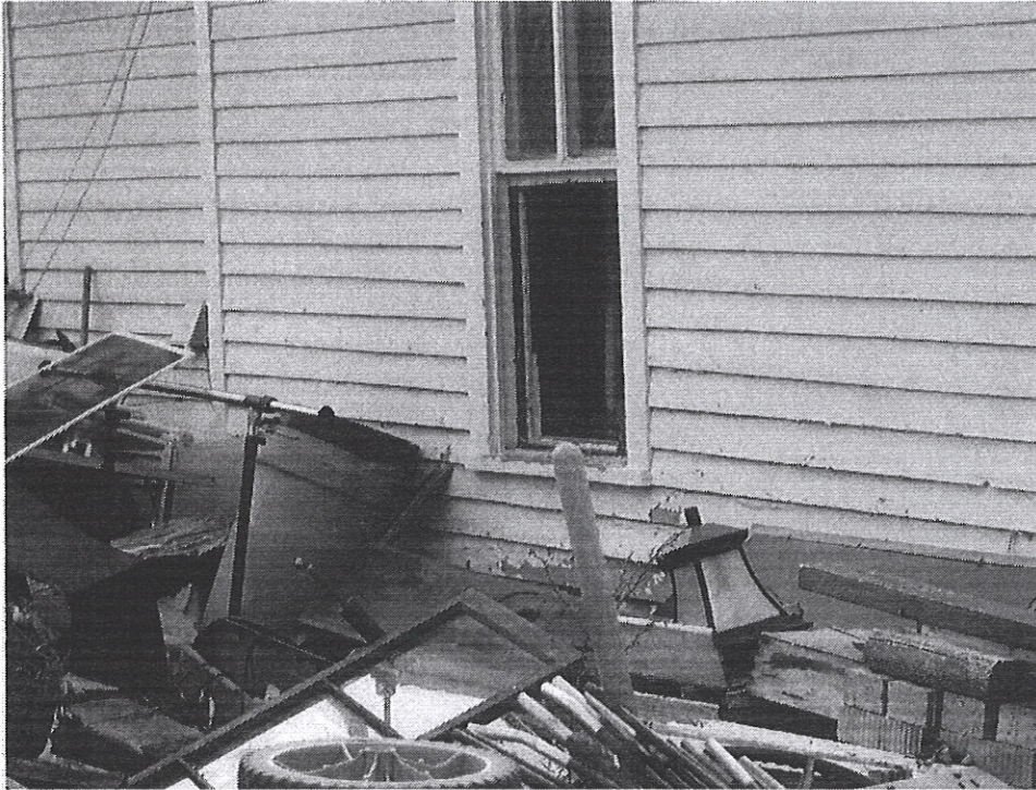
Broken Window on east side of house
