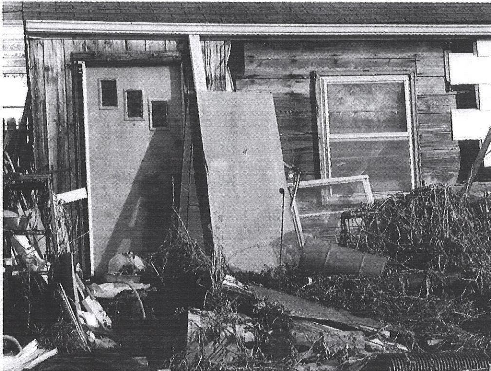
Siding missing on garage
