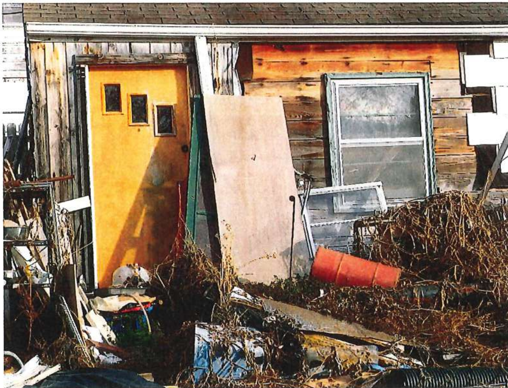
Siding missing on garage
