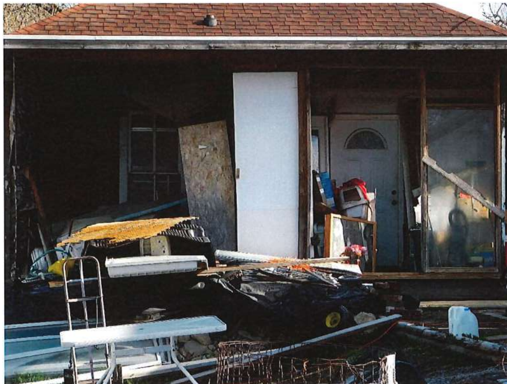
Bottom: siding missing on garage. This area still has accumulated items that need cleaned up.
