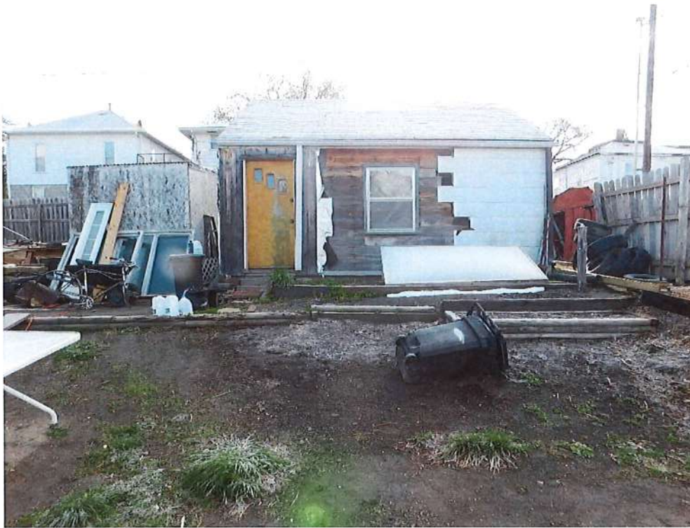
Top: siding missing on garage
