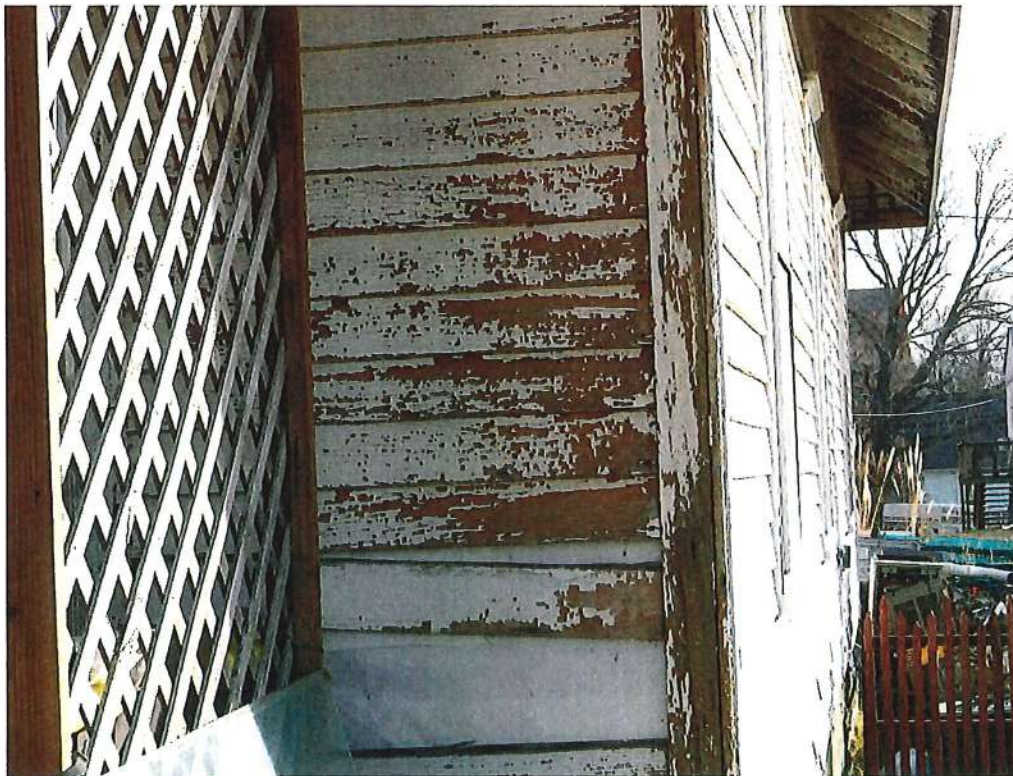
Paint peeling on North side of house and under eaves
