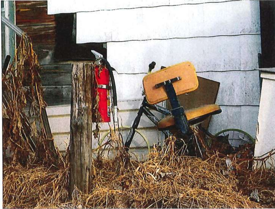
Siding missing on the garage.
