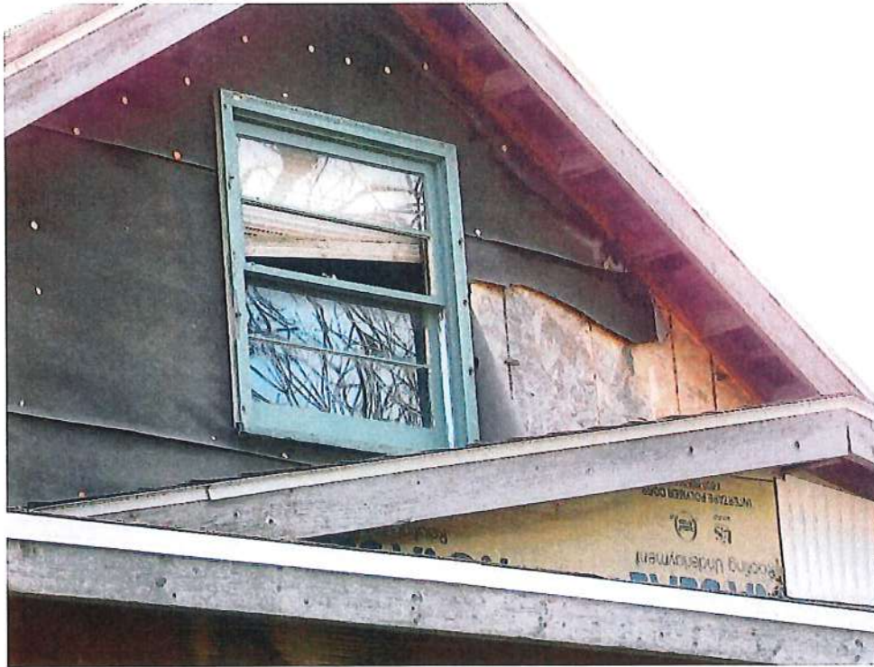
Broken window and missing siding north side of house
