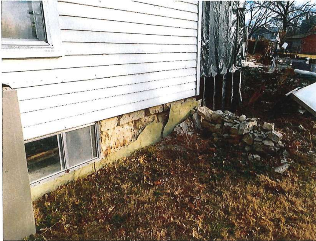
Southwest corner of the house. Mortar is missing between limestone blocks
