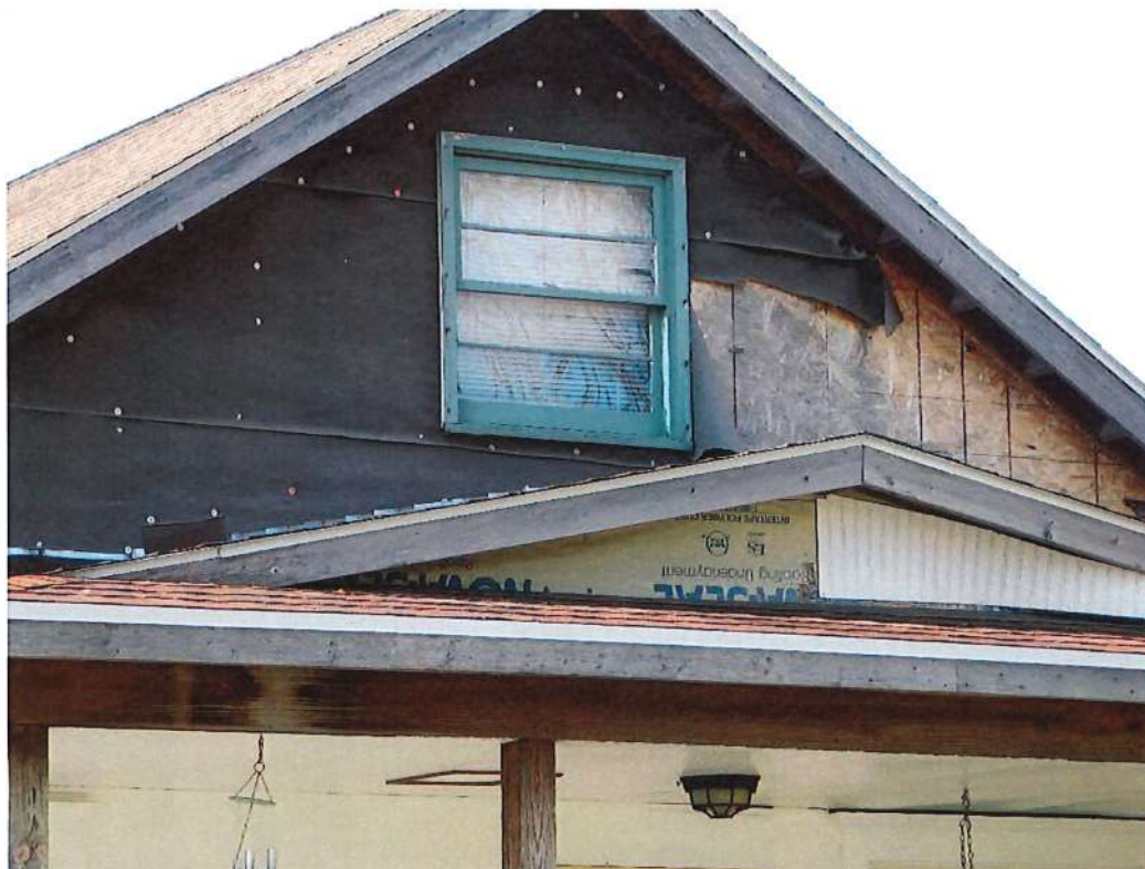
Bottom: Window fixed. Siding still missing
