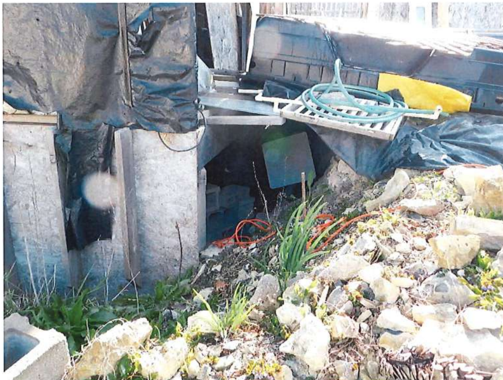
Back porch: foundation under porch not repaired. Dirt work not done to make ground slope away from porch.
