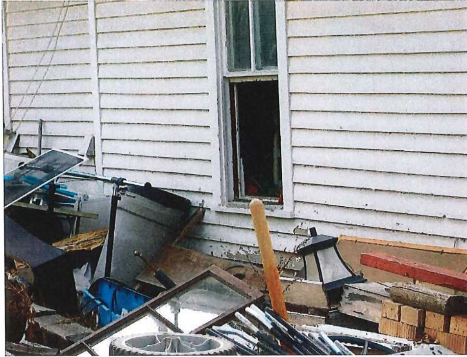
Broken Window on east side of house
